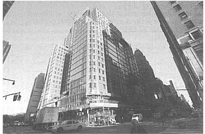
1775 Broadway; the value of New York metropolitan area office buildings is down 40 percent from its peak in late 2007.
